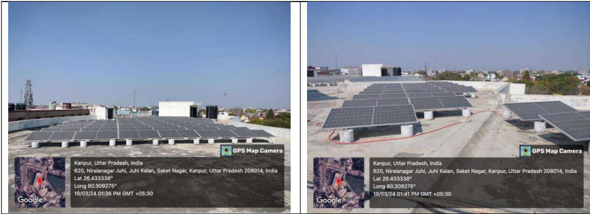
K1.Solar Power panel
