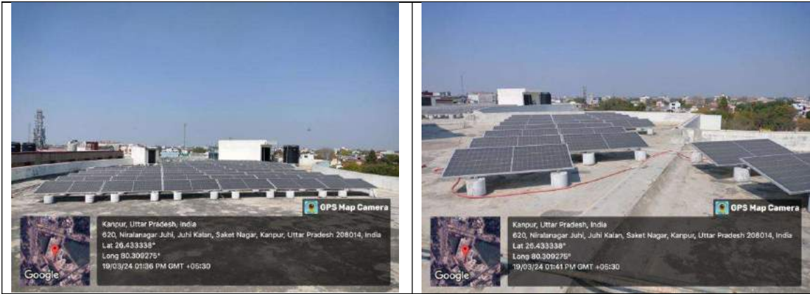
K1.Solar Power panel
